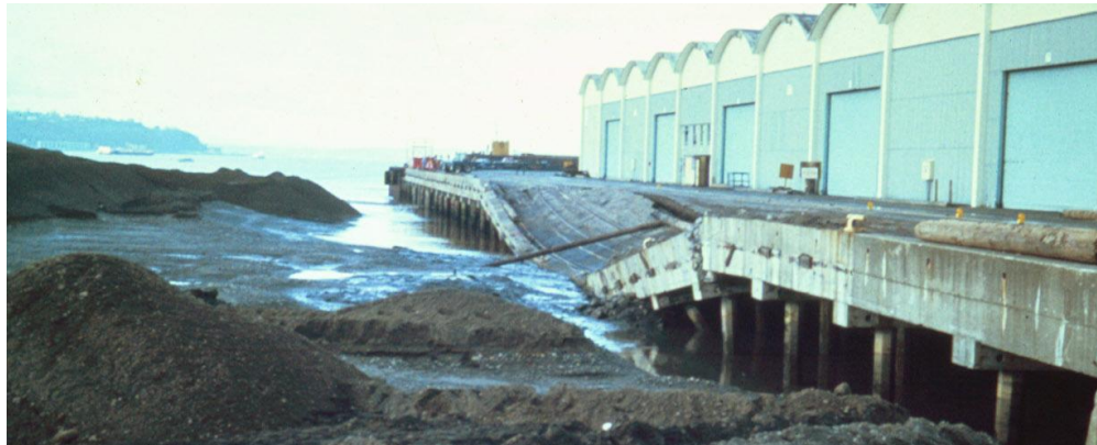
Fig. 7.51 View of the consequence of a hydraulic fill of fine silt flowing against 24-inch piles.
