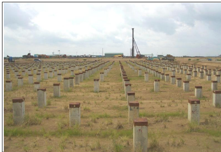
Fig. 15 View on October 4, 2011, from south end of CFS building showing some of the about 750 piles driven for the CFS building (Authors' photo)
